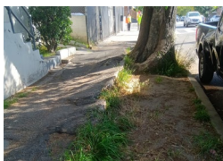
Tree roots lifting sidewalks
