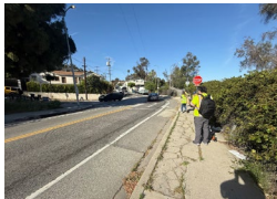
Cracked and narrow sidewalks
