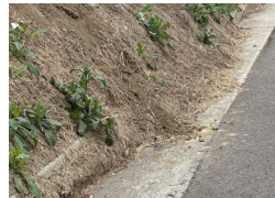
Hillsides overflowing onto sidewalks
